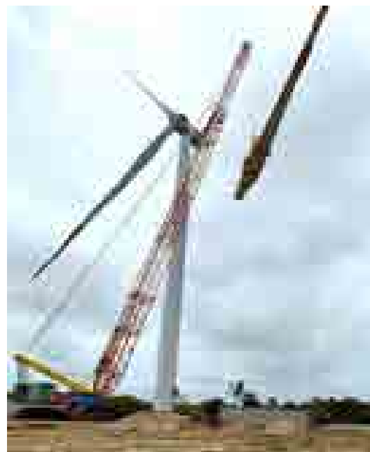
Figure G3: Upgrading the Blade Lightning Protection system at Thambapavani Wind Power Station.
