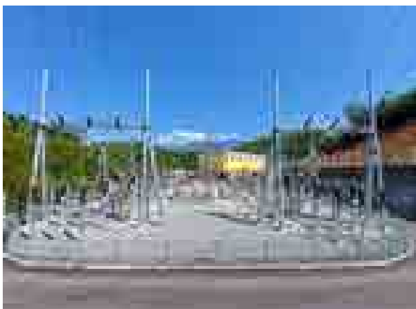
Figure P1: Broadlands Power Station Switch Yard
