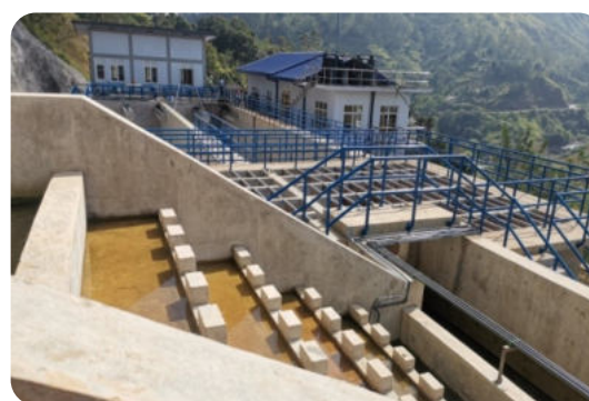
Ettampitiya Water Treatment Plant
