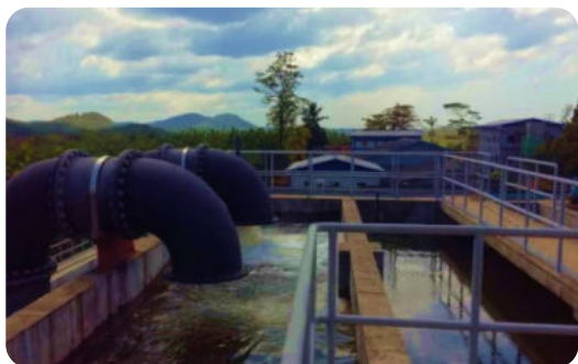
Water Treatment Plant - Kethhena
