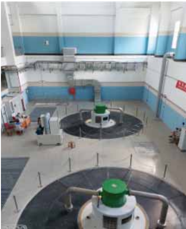
Figure P2: Broadlands Generator Floor
