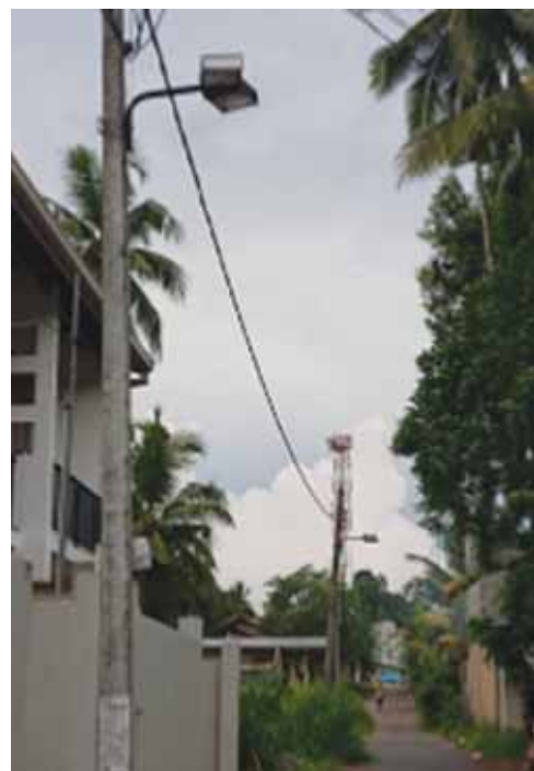
Figure C1: Energy efficient street lighting
