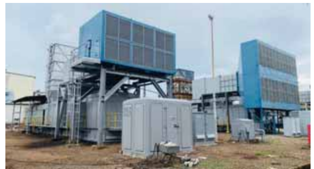
Figure G5: Rehabilitated frame V gas turbines
