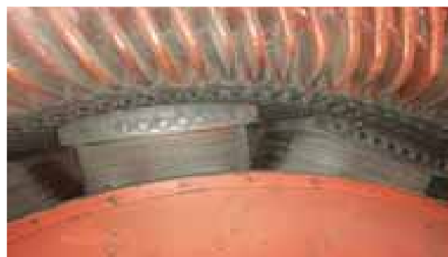
Figure G2: Unit 4 Generator at Old Laxapana
