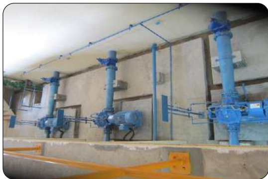
Kandana Pump House
